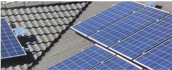
Any inter-array cables are hidden.
