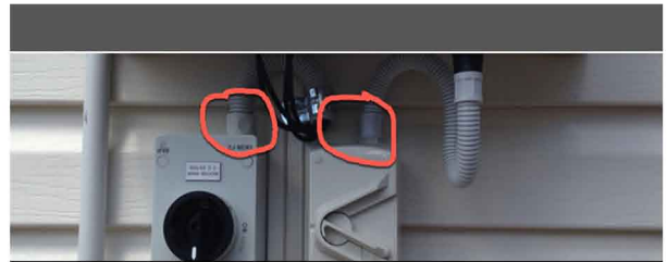
Top entry into DC isolator
