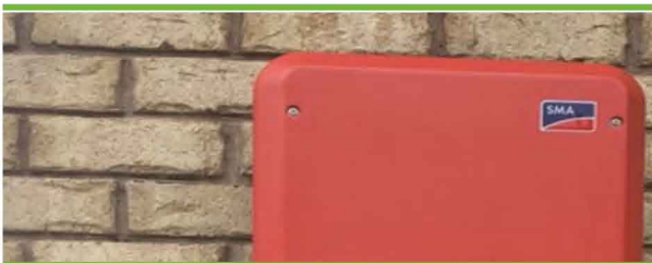
Bottom entries into the isolator
