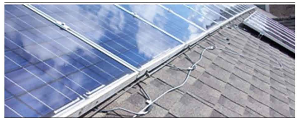
Cables are not done under the roof
