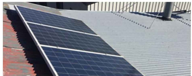
Panels not aligned
