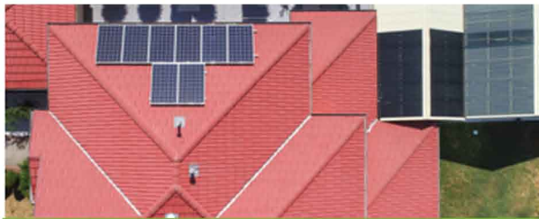
Cables and conduit under the roof. Aligned panels
